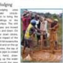
Hand-dug well with concrete lining
