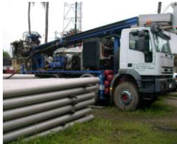
Figure 8 Stainless steel screens and new rig in Lagos
