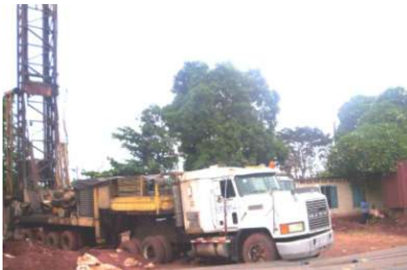
Figure 6 A heavy duty rig imported from the US capable of drilling to 1500 m depth
