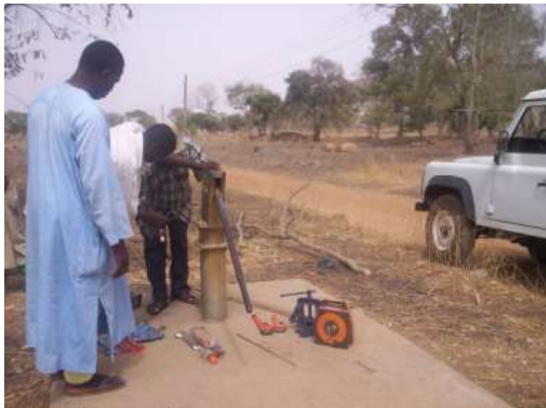
Figure 11 A non functional handpump under repair
