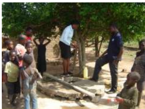
A private well in Amuria district. Deepened, brick lined and covered on top in preparation for a hand pump
